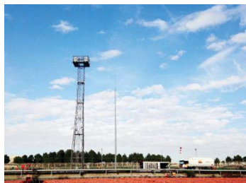
HIGH MAST LIGHT
